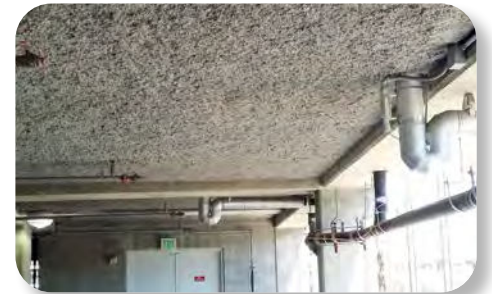
Insulseal shown in gray; Omni Hotel Cowboys Practice Facility, Dallas, TX.
